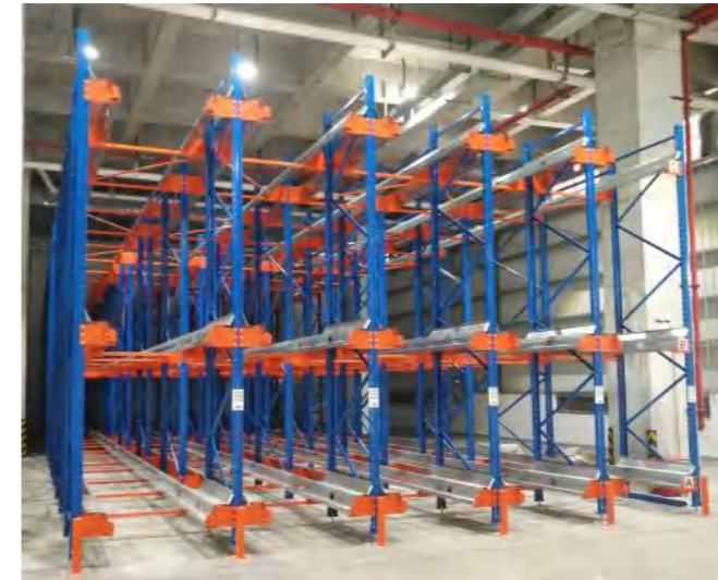
Radio shuttle rack project 穿梭式货架案例
