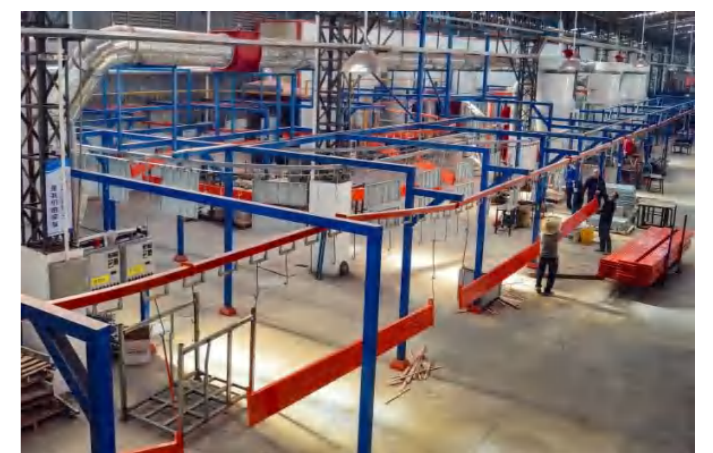
Painting line 喷涂线
